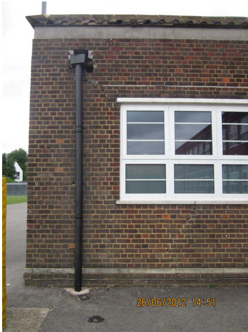
Figure 2- Stepped Cracking Outside Sixth Form Common Room
