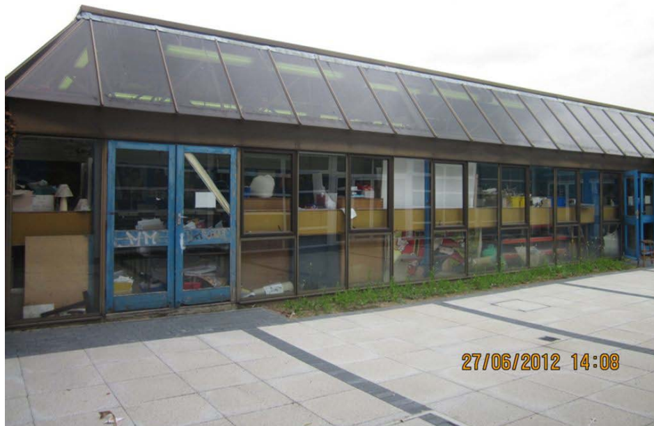
Figure 4- External Timber Doors in Poor Condition
