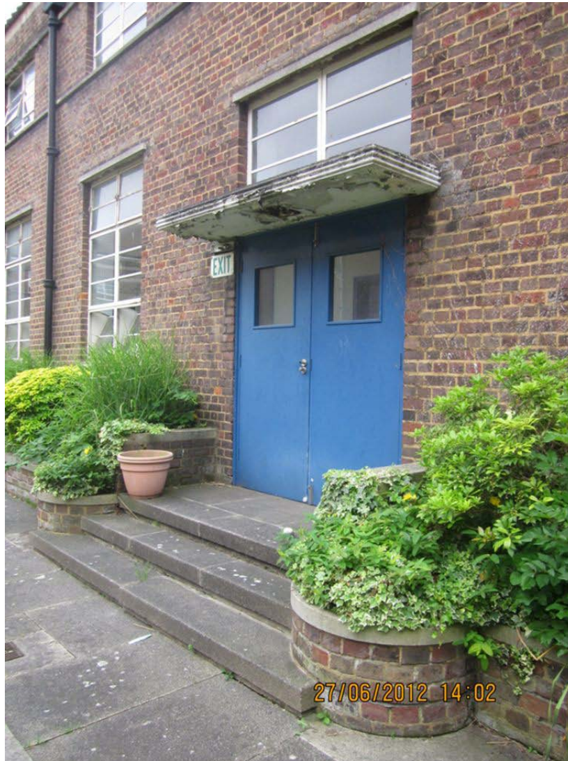
Figure 5- Defective Concrete Canopies
