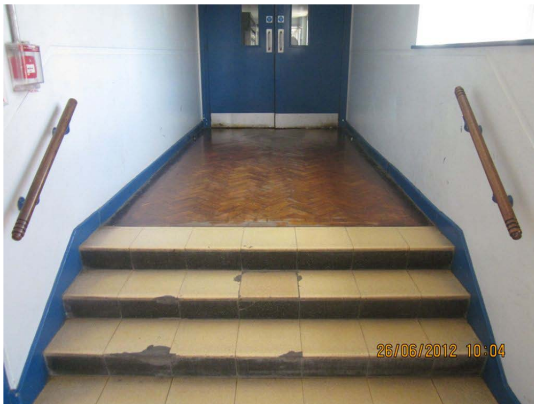
Figure 6- Poor Condition of Floor Coverings to Stairs
