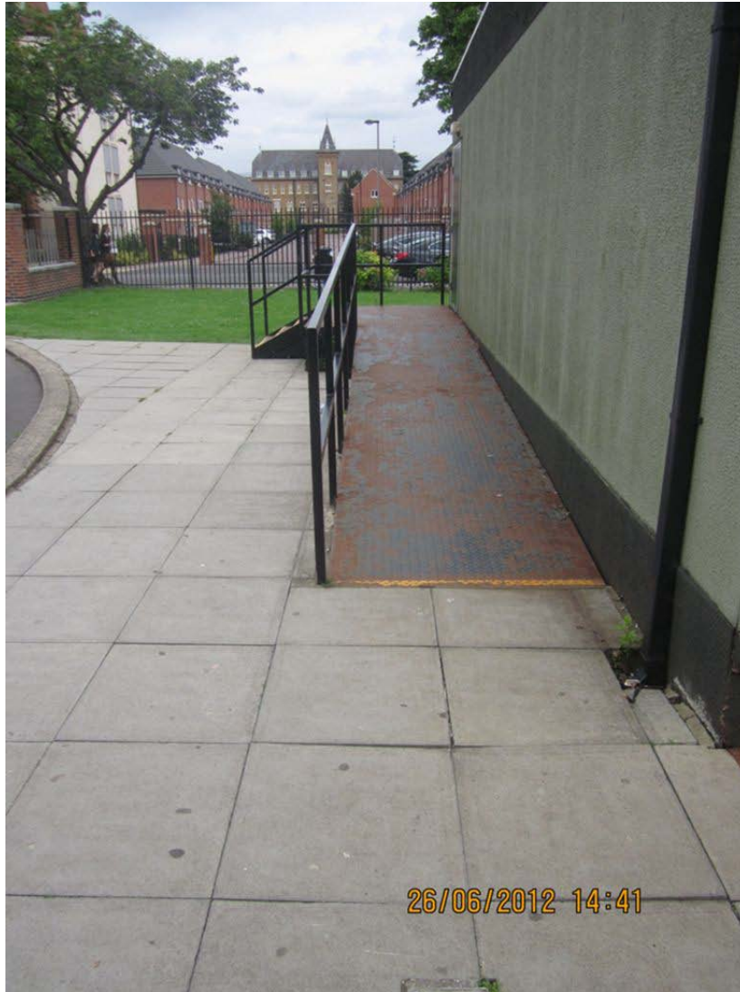
Figure 9- Corrosion to Access Ramps
